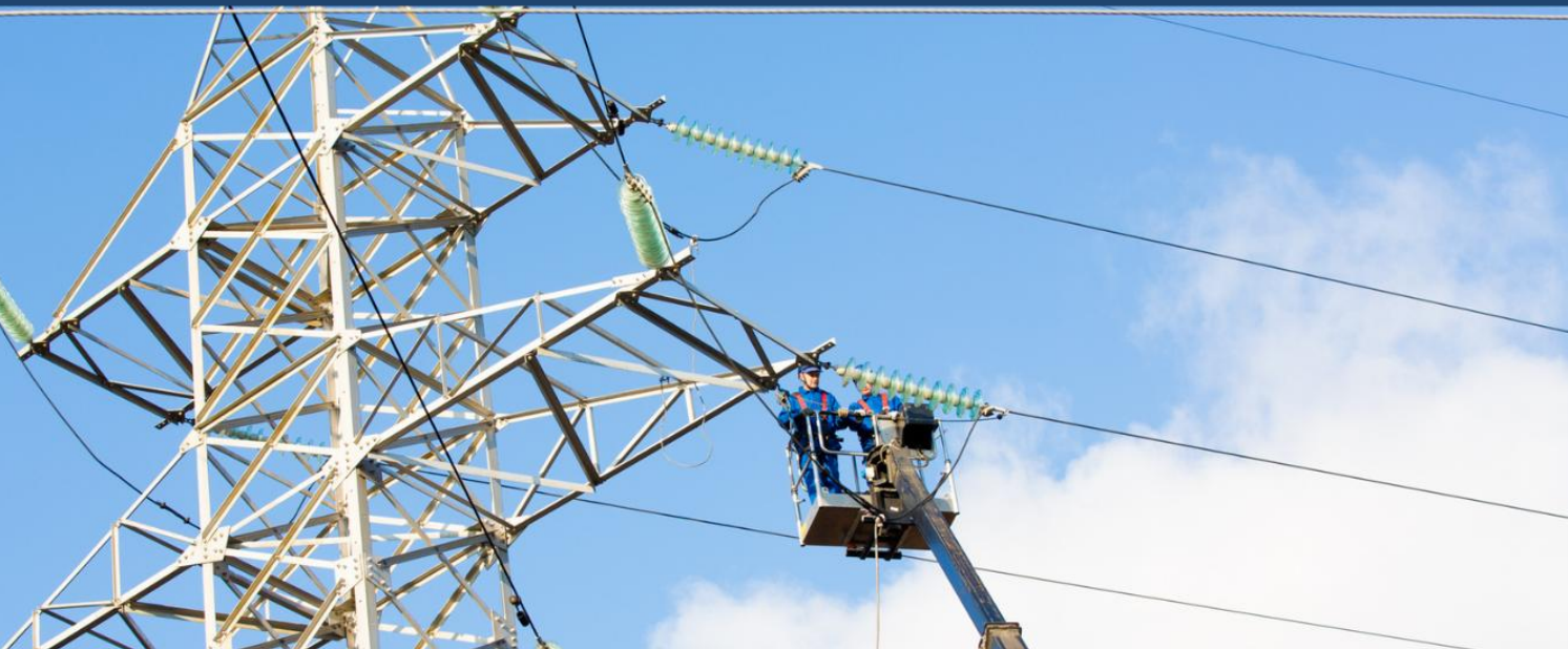
Premier Energy's electricity distribution network in the Republic of Moldova.
