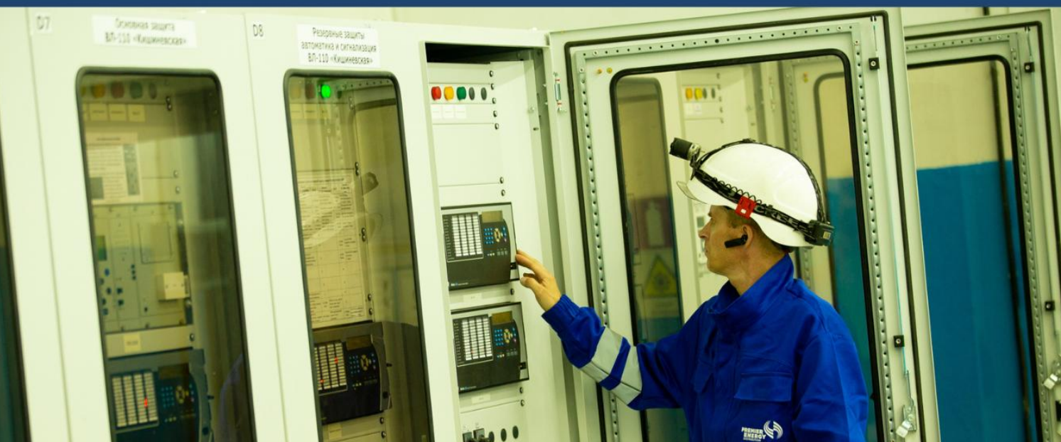
Premier Energy's electricity distribution network panel in the Republic of Moldova.
