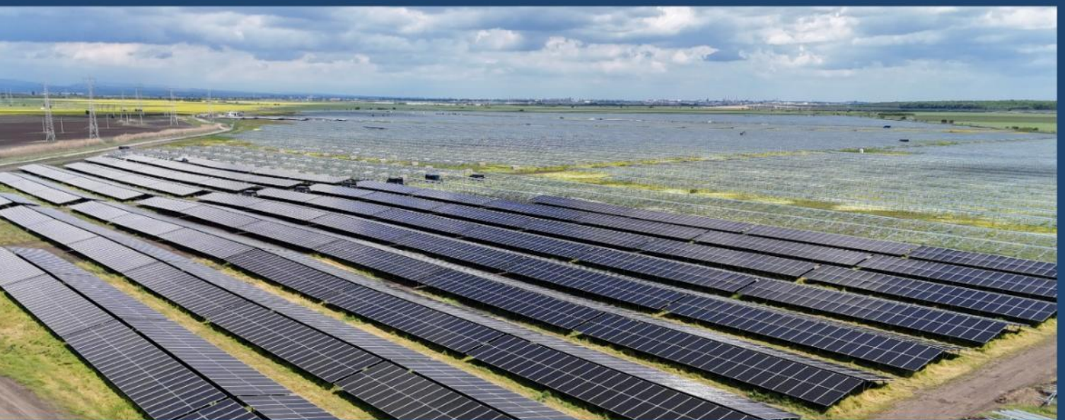
Premier Energy's 48 MW solar park development with 16 MWh battery storage capacity currently under construction in Buzau county, Romania.
