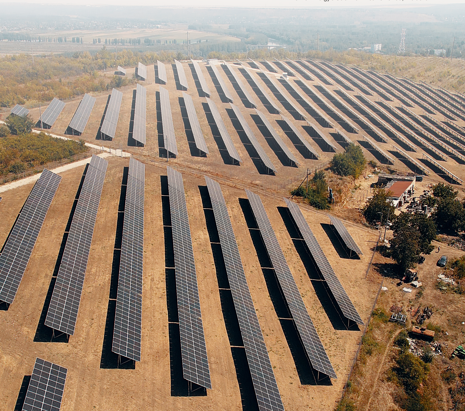
Premier Energy's Solar Park near Chisinau, Moldova
