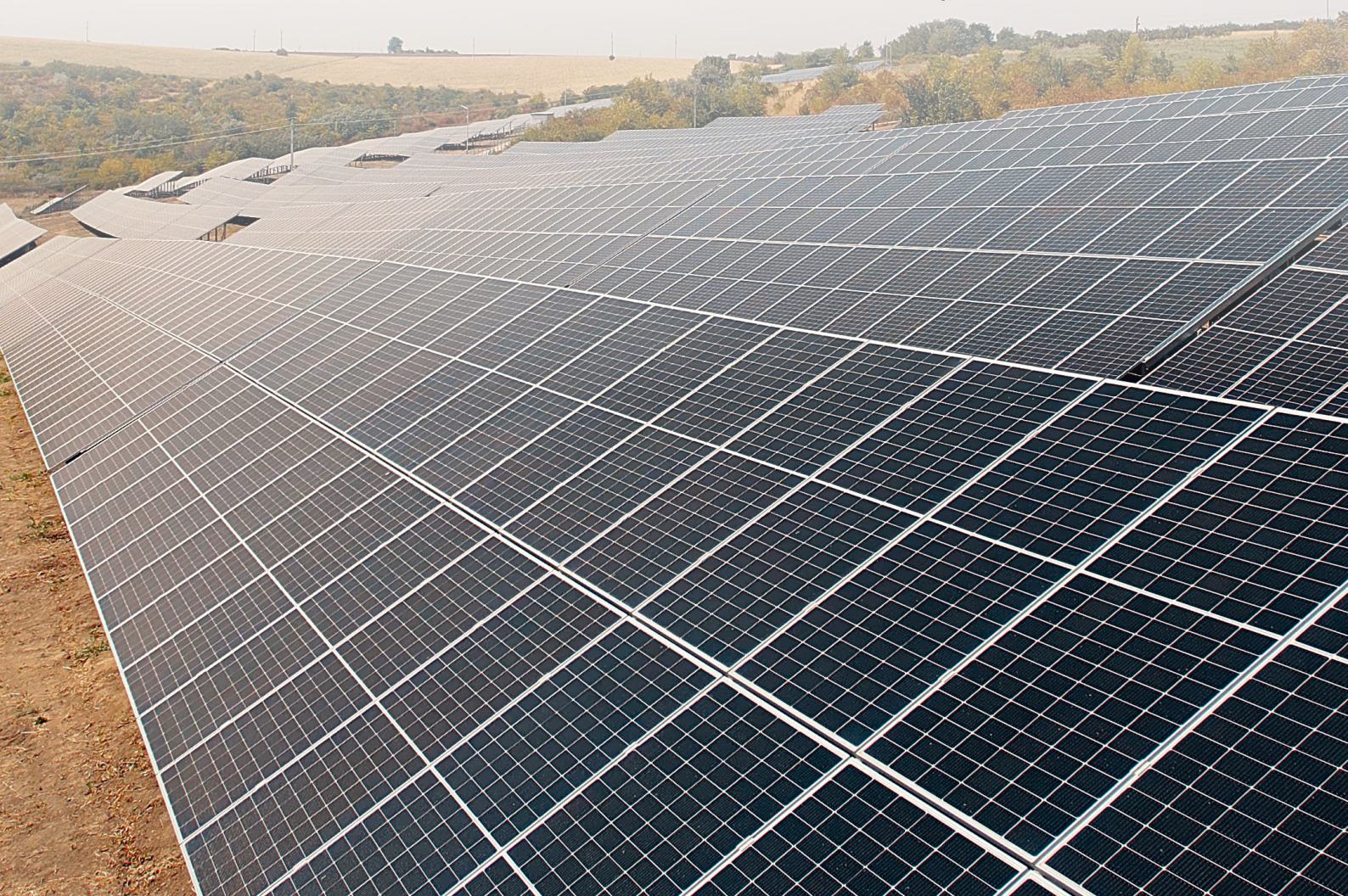
Premier Energy's Solar Park near Chisinau, Moldova
